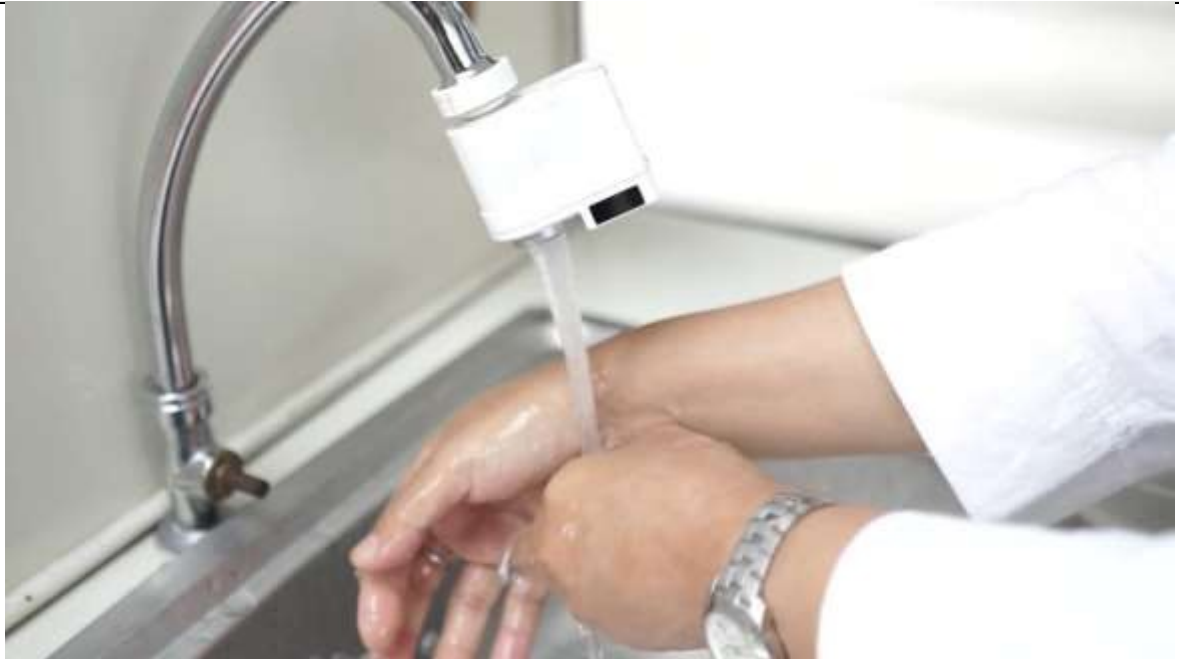
Sensor Water Faucet in Central Administration Building
