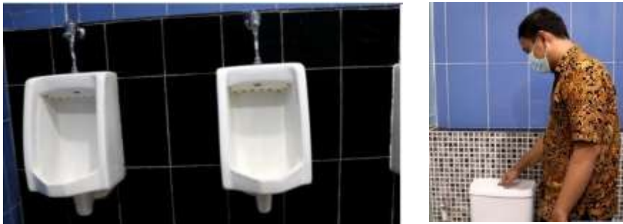
Use of urinal flushing system and toilet flush in the Faculty of Pharmacy
